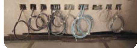
The view of a row of outlets will be disguised by an additional joinery facade
