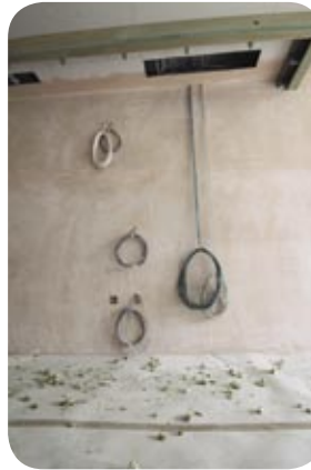
Varying levels of cable outlets include Cat.5 for phone and data at the bottom and at midlevel for an iPod docking station. The highest cabling is to power and control lighting under fitted cupboards
